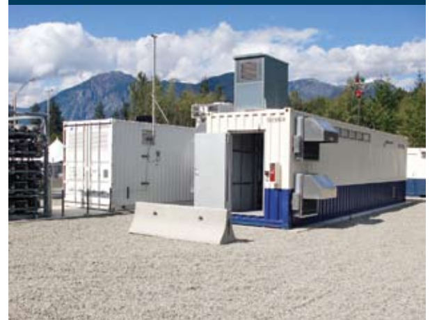
Renewable power system at Bella Coola, Canada.
