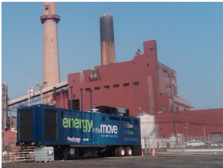
Figure 3: 1MW CLEARgen™ system installed at FirstEnergy
